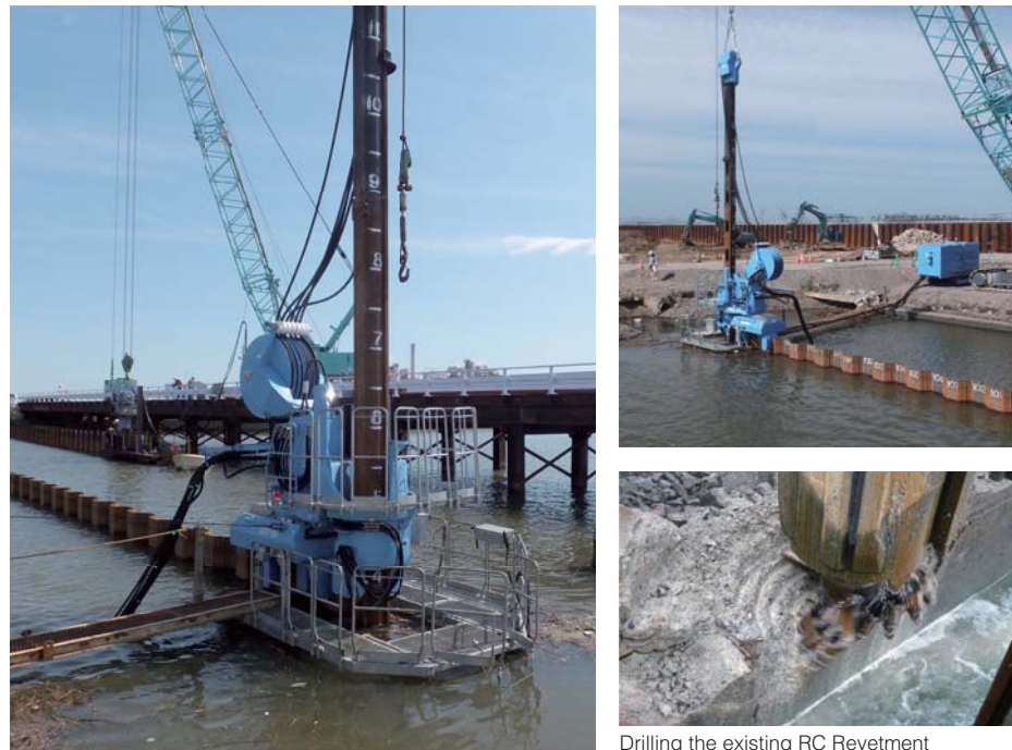
Project : Embankment Restoration Work Section 4, Natori River Location : Natori City, Miyagi Period : September 2013 ~ October 2013 Silent Piler : F201 Type of Sheet Pile : U Sheet Pile SP IIIw and SP IVw Pile Length : 7.5 ~ 16.5 m
