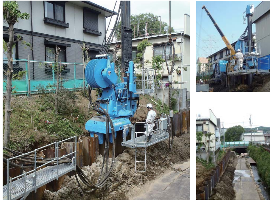
Project : Machida City Public Sewer System, Storm-Water Sewer Construction Works Location : Machida City, Tokyo Period : May 2013 Silent Piler : F201 Type of Sheet Pile : U Sheet Pile SP VL Pile Length : 8.5 m
